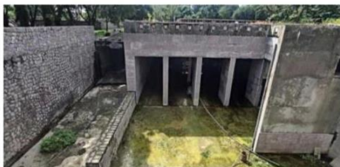
The nearly finished interpretation centre at the Qutb Shahi Tombs complex that is getting weathered due to disuse.
